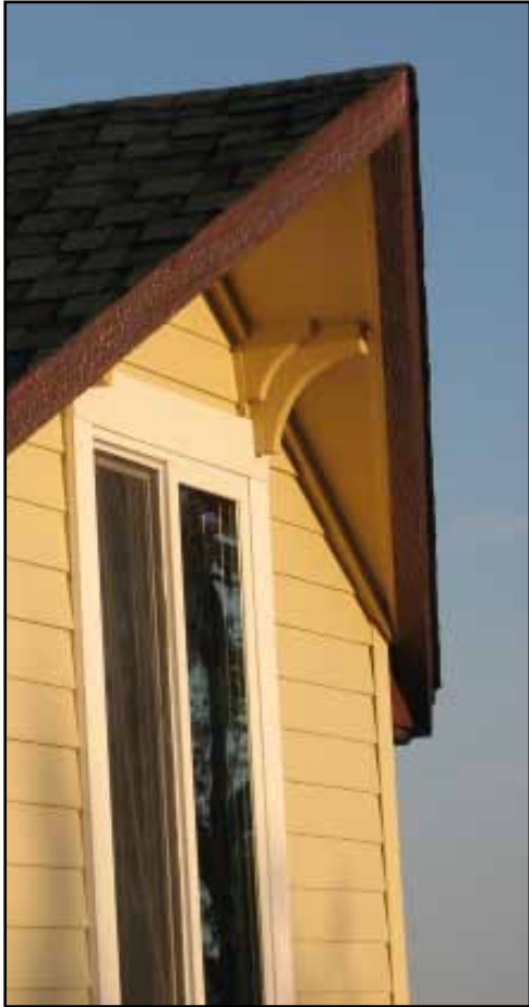
Existing homes can and should be made fire resistant too.
