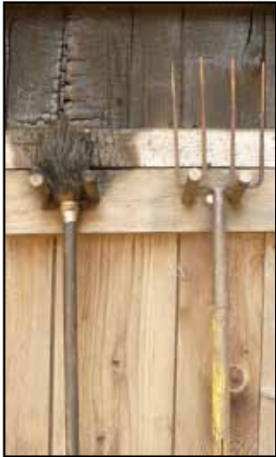
Though it charred the siding, luckily, the broom didn't fully ignite this building.
