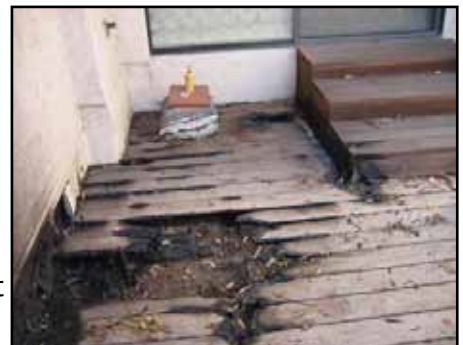
Consider replacing ground level wooden decks with non-combustible patio materials such as brick, stone or concrete.
